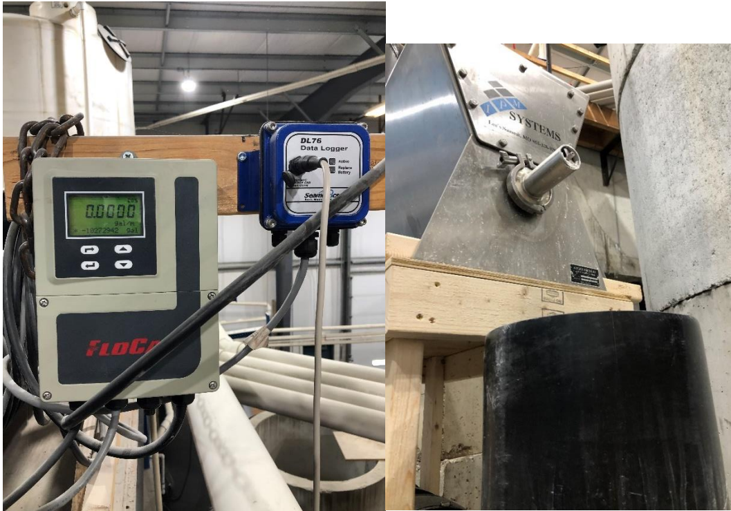
Figures 4 and 5 Photographs of Flow Meter and Sediment Delivery Port
